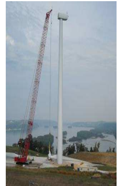
Turkey Hill Wind Project
