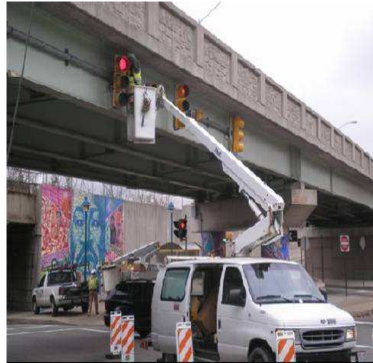
Turtle Creek Lighting Retrofit Project
